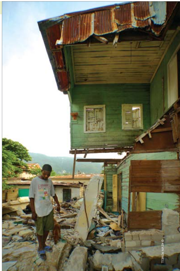
A concrete addition to this wood-frame house crushed and buried this man's cousin.
